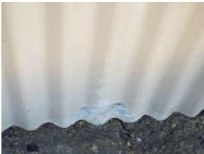
small area of surface rust needs treating at the front of the house
